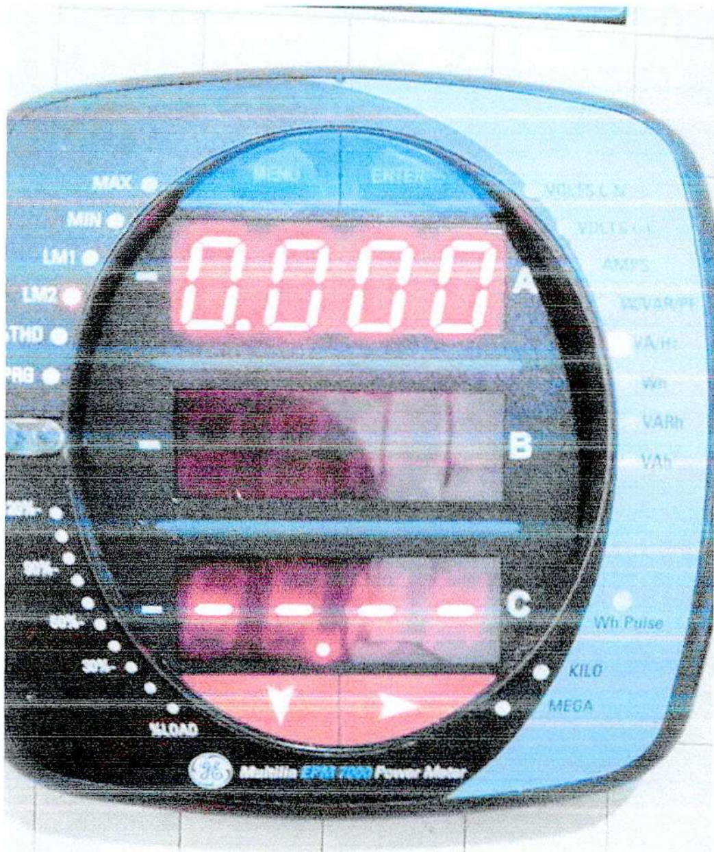
Item No. 10_Multimeter_Electro Industries Gauge Tech Shark 100
