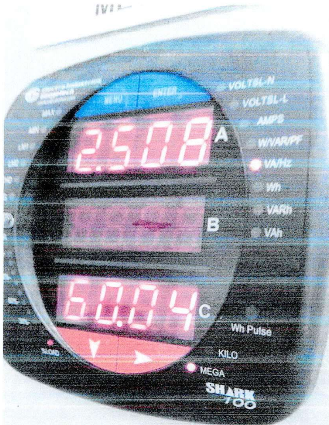
Item No. 10_Multimeter_Electro Industries Gauge Tech Shark 100
